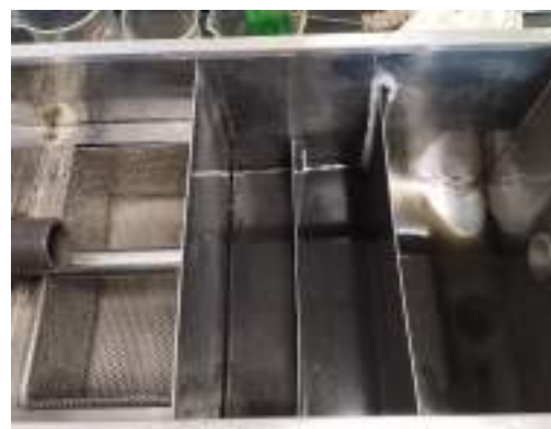
Plates 3. 2 Restaurant Wastewater in Modified Grease Trap
